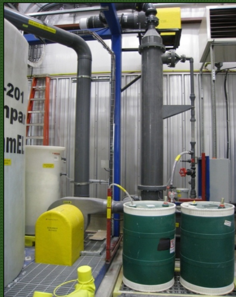
Chlorine Gas Scrubber
